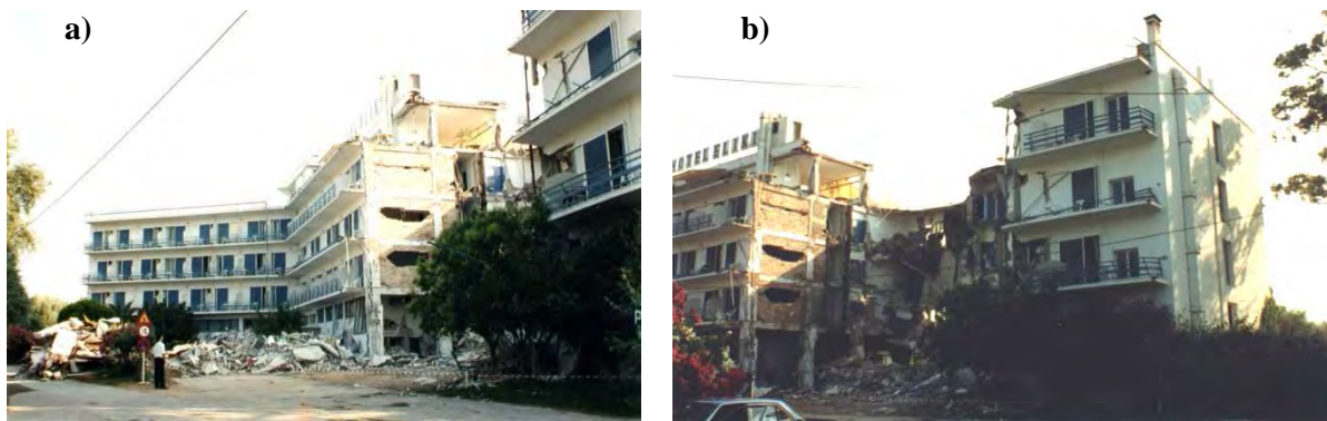
Figure 9: Typical example of partial collapse of buildings after the Egion 1995, M=6.7 earthquake. The rest of the building suffered limited damage, [16], [17].
